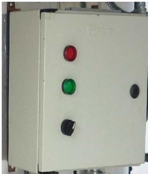
FIGURA 6-12: Tablero de control
