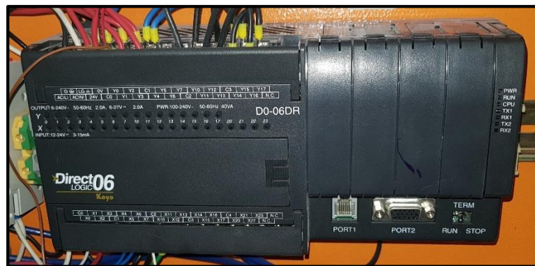
Figura 21. PLC Koyo Direct Logic 06
