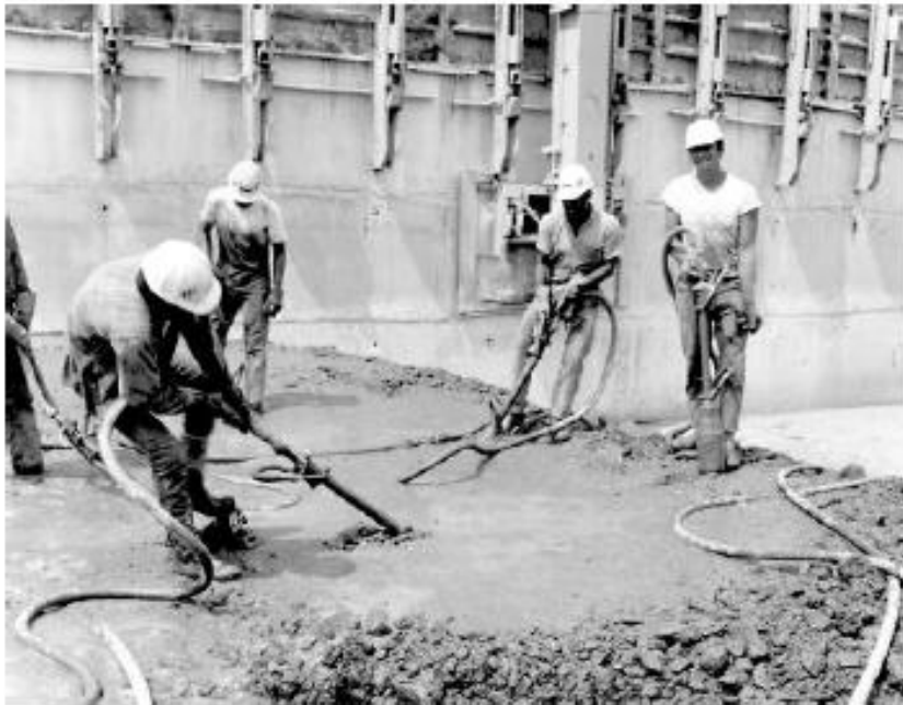
Fig. 7.6.1(b)—Haphazard procedure may result in mortar accumulation at the surface and leave rock pockets below, particularly at batch perimeters
