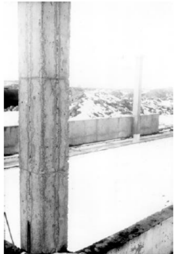
Fig. 6.4—Sand streaks caused by mortar leak
