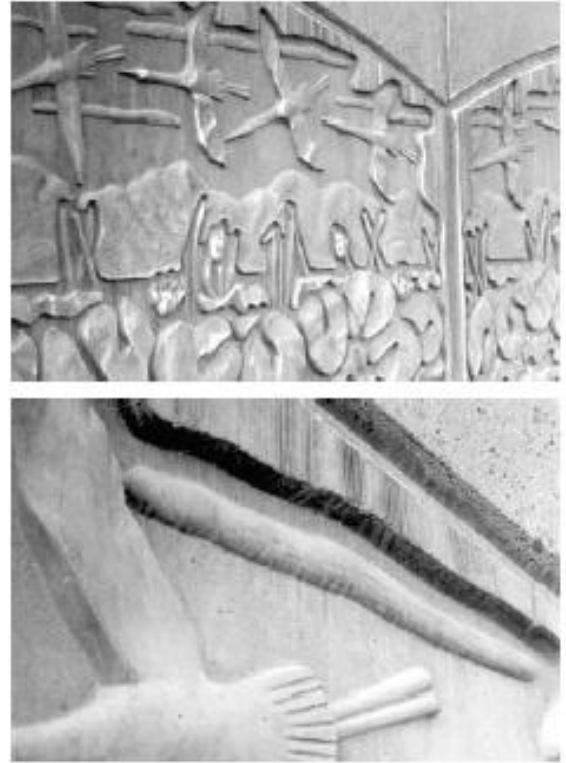
Fig. 1(c)—Close-ups of surfaces resulting from good consolidation
