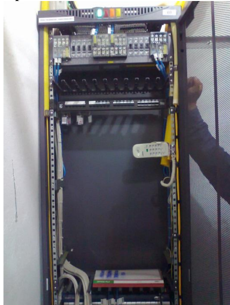
Optical Distribution Frame
